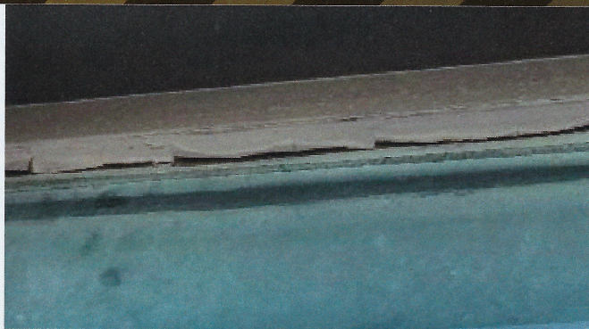
Delaminating paint visible
