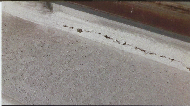
Standing water painted over on windowsill
